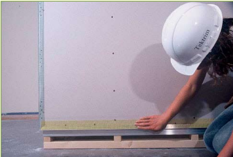
Figure 5-10: Apply screen tape or paper tape to the joint between the drywall and the UMB.
