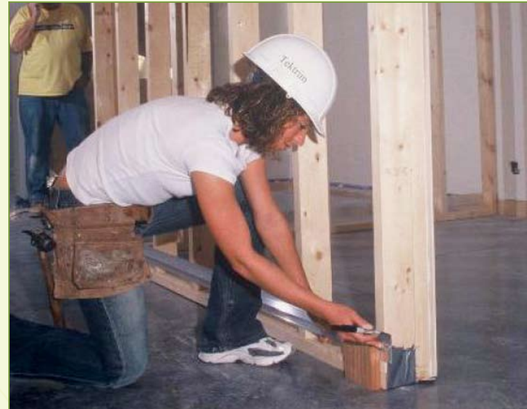
Figure 2-3: Cut square blocks to the dimensions of your UMB height and position the UMB on the floor resting on these gauge blocks.
